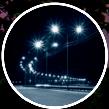
Street Lighting, High Mast & Poles
