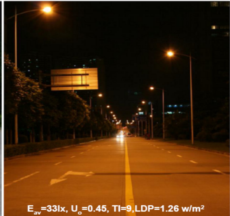
Street lighting with 250W HPS lamp
